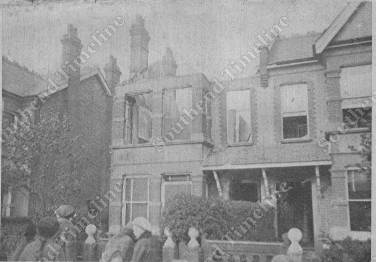
1. Butcher's Shop Damaged in Hamlet Court Road.
